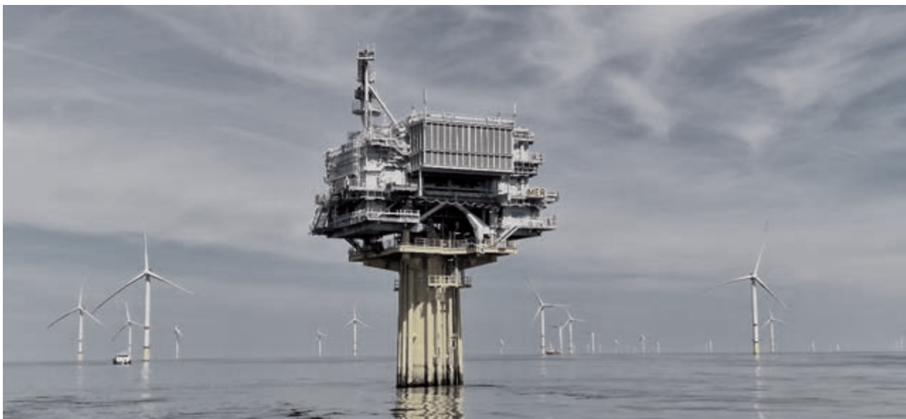
SLIKA 2: OFF-SHORE PLOŠČAD, OSS MERMAID, BELGIJA, SEVERNO MORJE, 2019, TRANSFORMATOR 1 × RT 260 MVA, 225/33 KV
